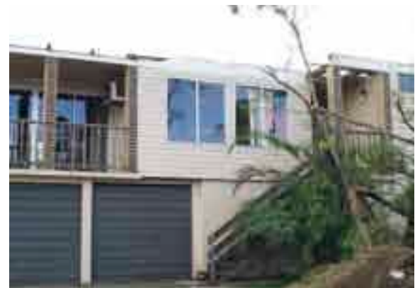
This house, marked with a red ‘N’ for ‘No’ was deemed uninhabitable by USAR crews.
