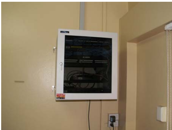
Figure 3. South office, data cabinet.
