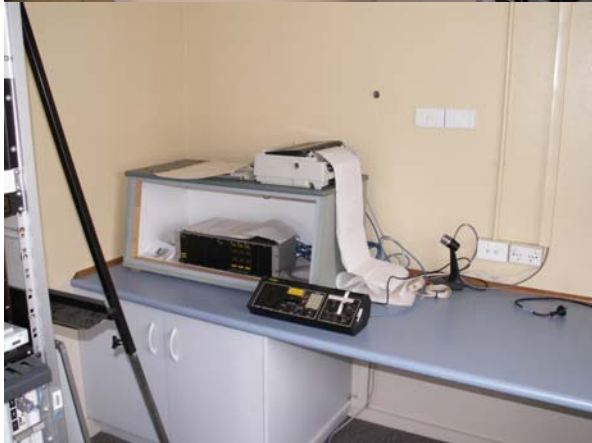
Figure 8. "Comms" room, "pico cell" and protected premises communication rack.
