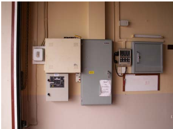
Figure 9. North-east corner, main appliance bay, switchboard.
